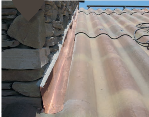
In the picture an example of incorrect installation.
