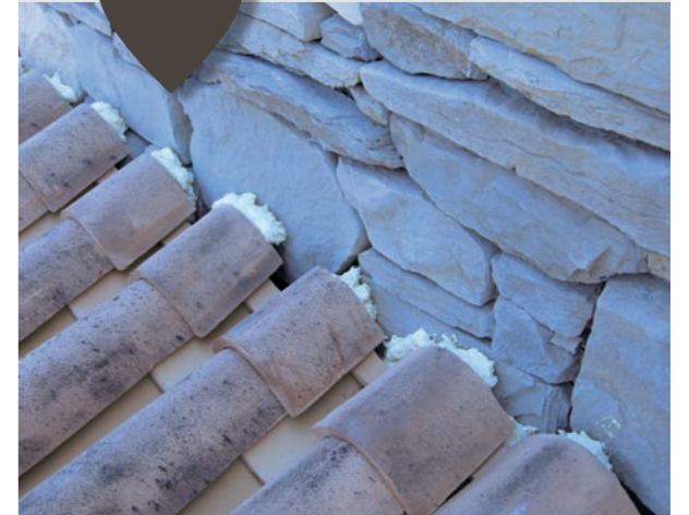
In the picture an example of incorrect installation.
